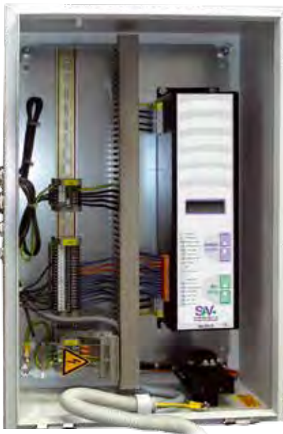
Control unit in switching box
